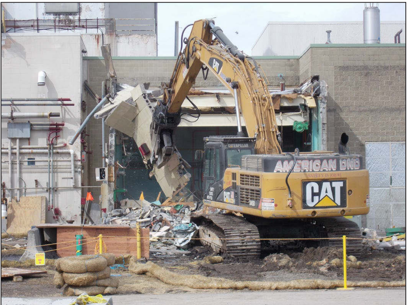
The West Valley laundry facility was one of seven ancillary support buildings to be demolished. Originally built in 1964 as the site's maintenance building, the support structure later became the laundry facility in the early 1970s. The 1,456-ft 2 building was constructed of concrete block, along with a steel frame and concrete slab on grade.
