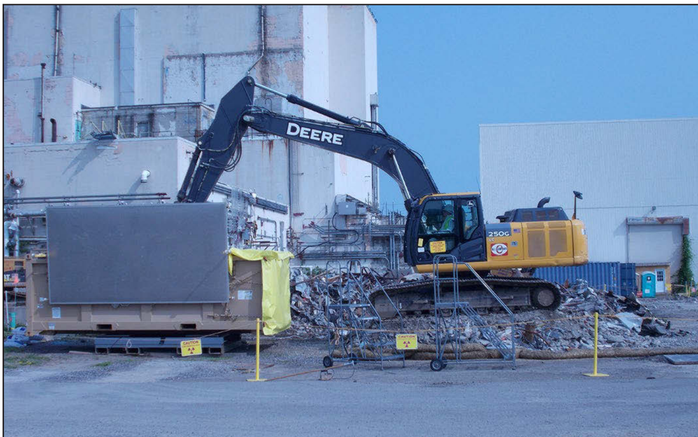
Debris from the demolition is loaded and packaged for off-site disposal. Scott Anderson, president of cleanup contractor CHBWV, said, "Protecting the workforce and the environment were paramount during the demolition process. We completed this challenging milestone using lessons learned and look forward to applying those best practices on future projects." ■
